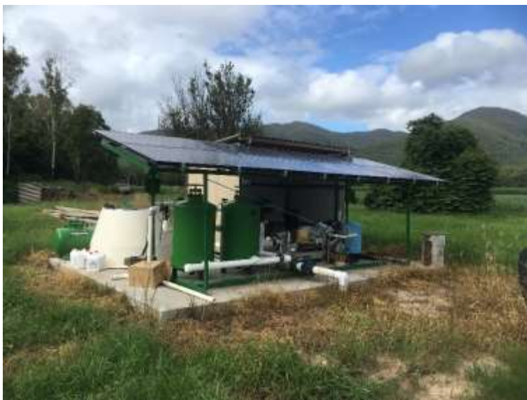
Figure 3 Trickle pump station
