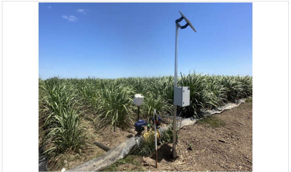
Timed actuator fully set up, with accompanying moisture sensor (G-dot).
